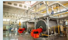
SITE, CITY BOILER ROOMS
